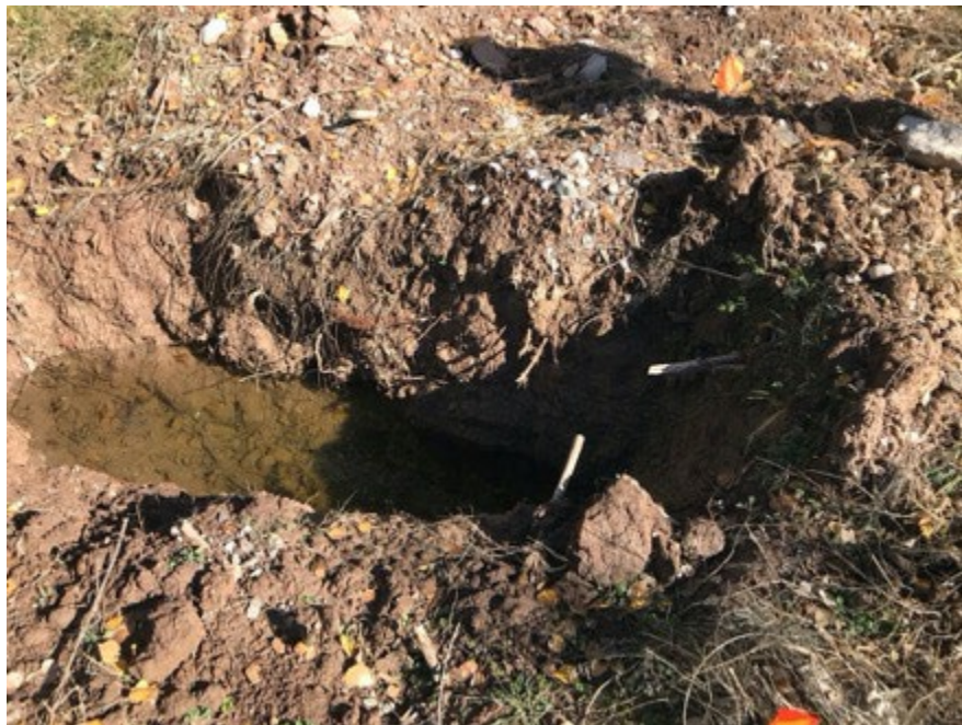
Photo 4. Hole dug in bottom of drainage near east end of Project showing ground water level.
