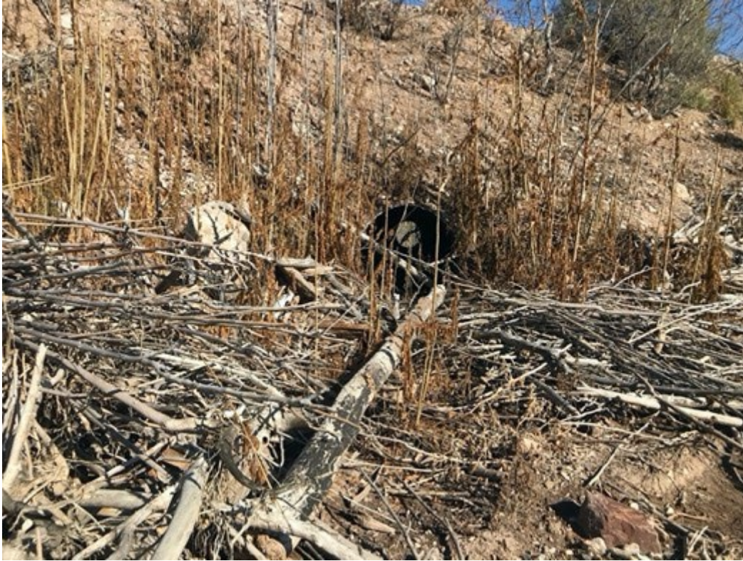
Photo 5. East end of project- terminates at entrance of culvert. Note young shoots of Tree of Heaven.
